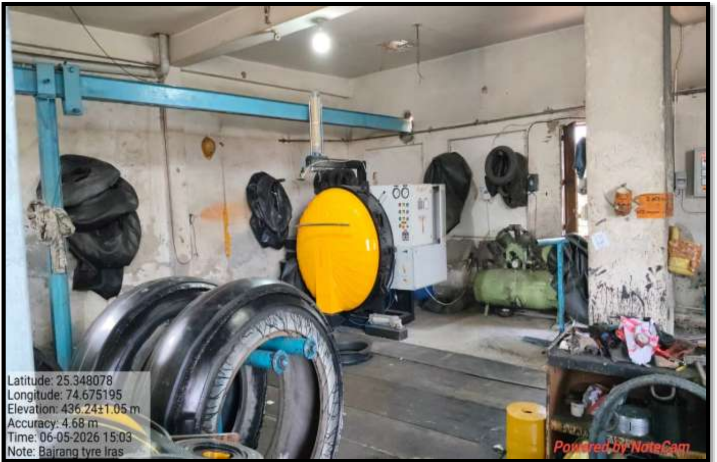
Figure 7 Electric Chamber for Tyre Retreading
