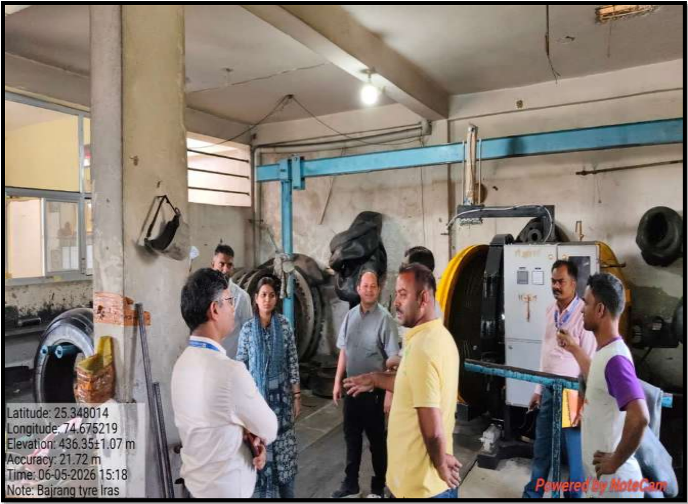
Figure 4 Committee Visiting Electric Chamber at M/s Jai Bajrang Tyre Retreading
