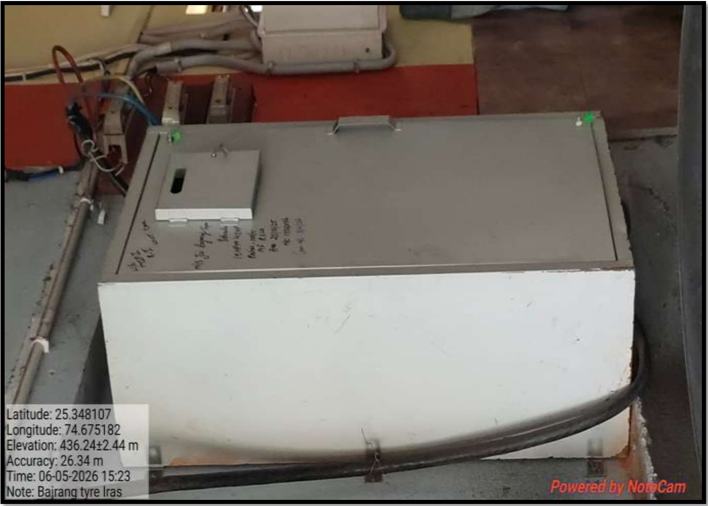
Figure 3 Electricity Connection at Jai Bajrang Tyre , Iras Road. Bhilwara
